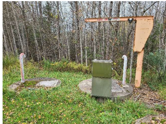
A picture of the Village's Lift Station wet well and valve vault. Upgrades to the Lift Station are included as part of the recommended alternative.
